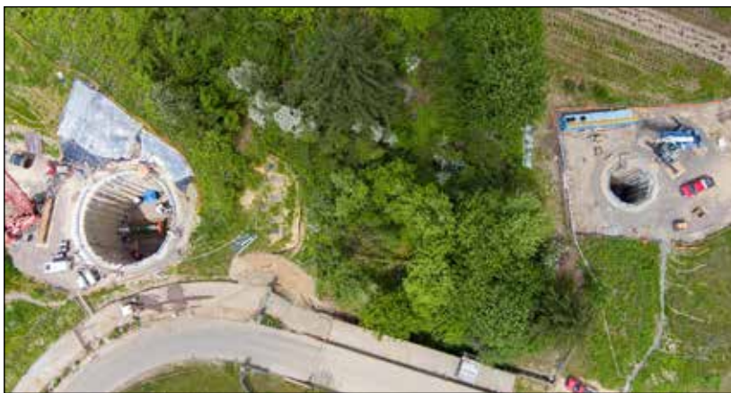
An aerial view of WWSP's trenchless crossing at Arrowhead Creek Park shows the sending shaft (at left) and receiving shaft (at right). The pipe ramming equipment is visible inside the sending shaft.
