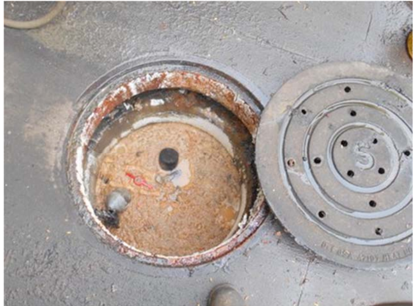
Grease in manhole
