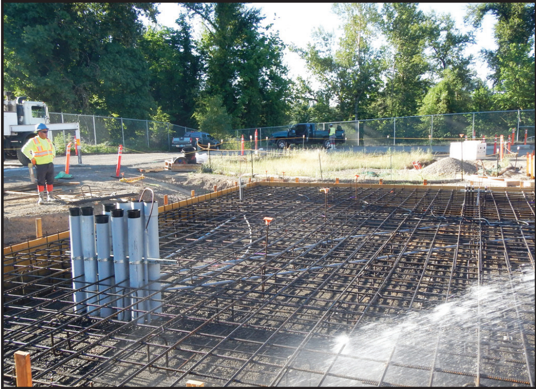
Foundation construction underway for the new generator needed to expand capacity of the Willamette River Water Treatment Plant (CIP #1144).
